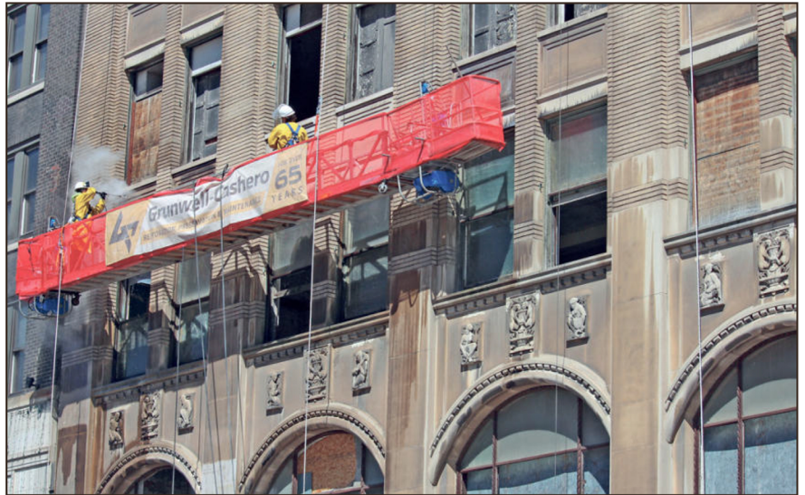
POWER-WASHING the 98-year-old brick and limestone exterior of the Park Avenue Building in Detroit are Laborer Rudy Leon and mason Tyler Tabor of Bricklayers and Allied Craftworkers Local 2. They're employed by Grunwell Cashero. The derelict building is getting readied for renovation after being empty since the 1990s.
